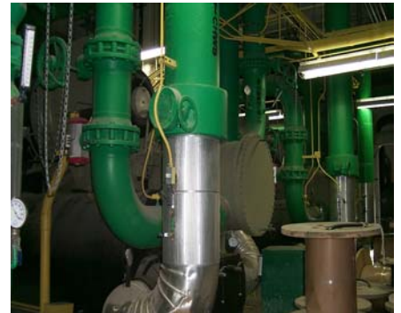
Row of four 1,000-ton chillers used to produce cold water for air conditioning throughout campus.
