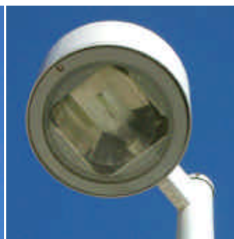
Parking lot fixture
